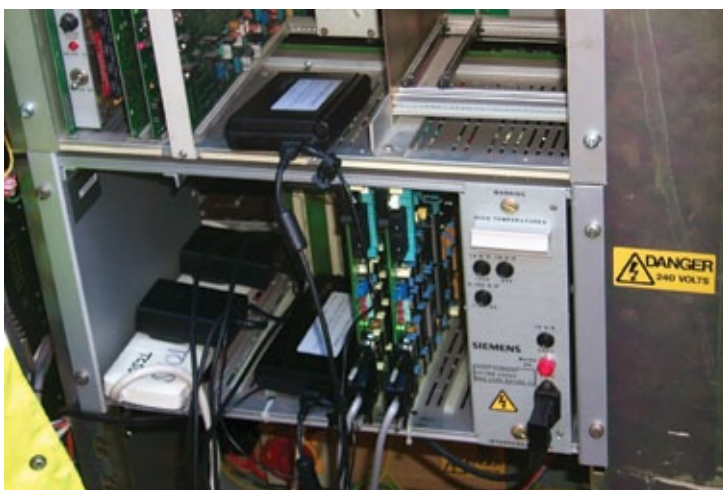
Bus priority module inside a roadside traffic signal controller
