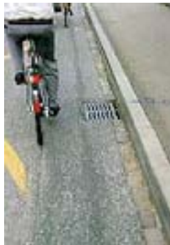
An "S" catch basin grid
